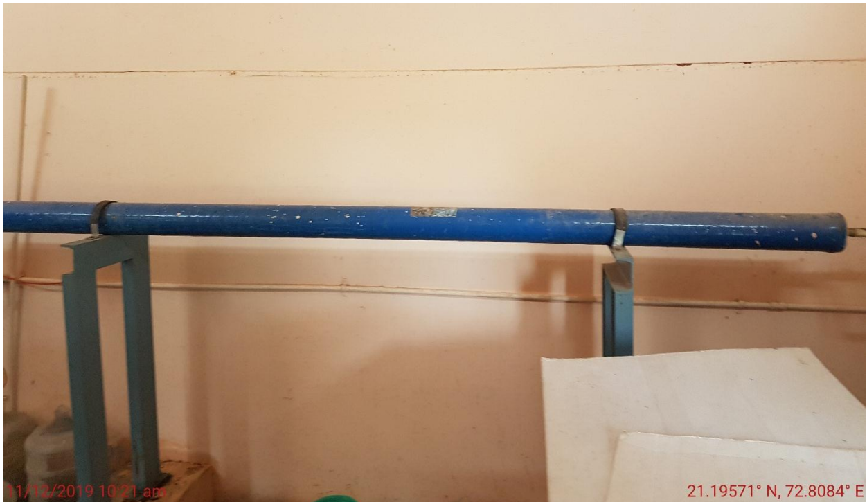
RO Plant of Capacity 750 LPH for Water supply in College Campus
