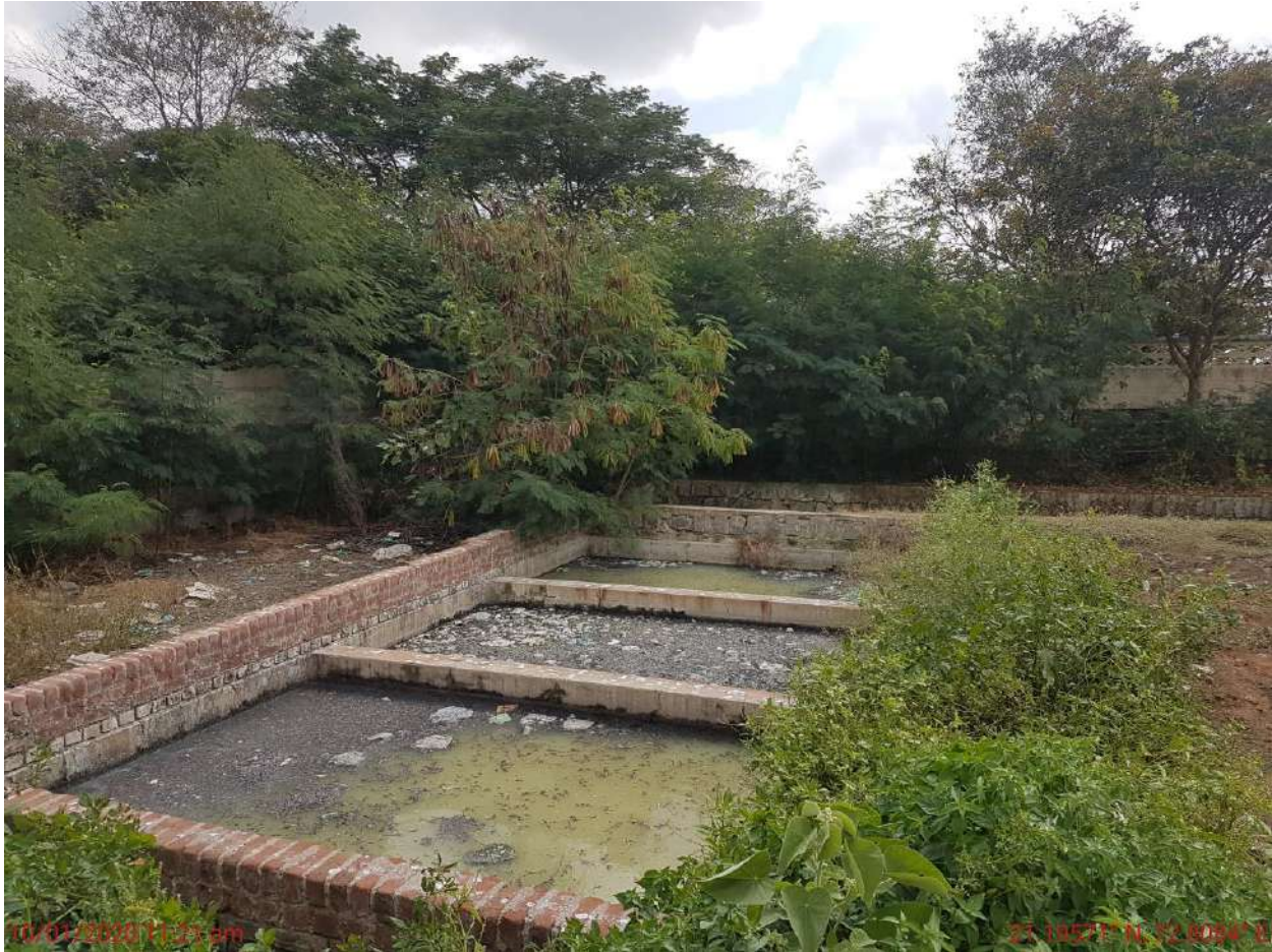
Sewage Treatment Plant of Capacity 50KLD
