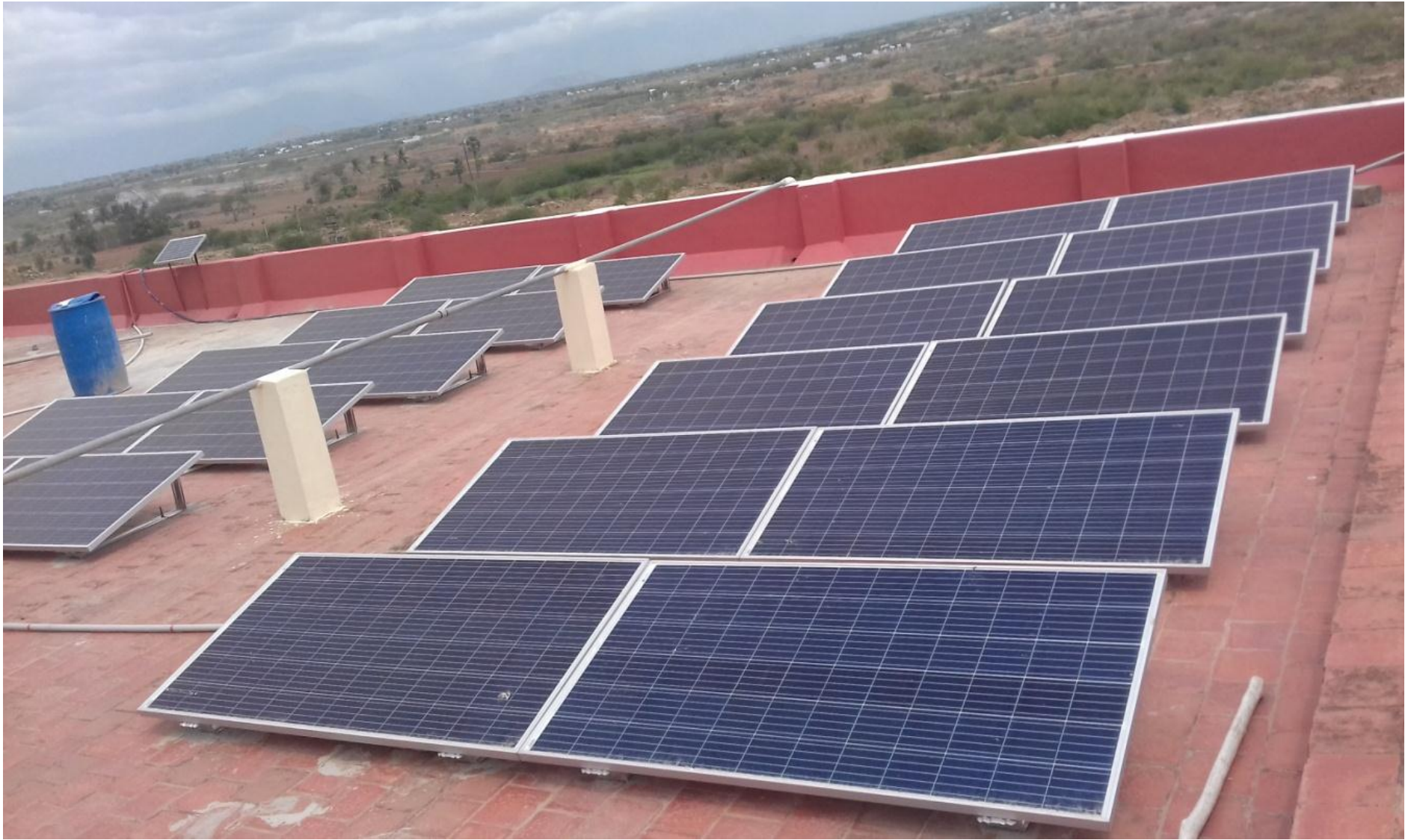
Solar panel placed in top of the EEE Department
