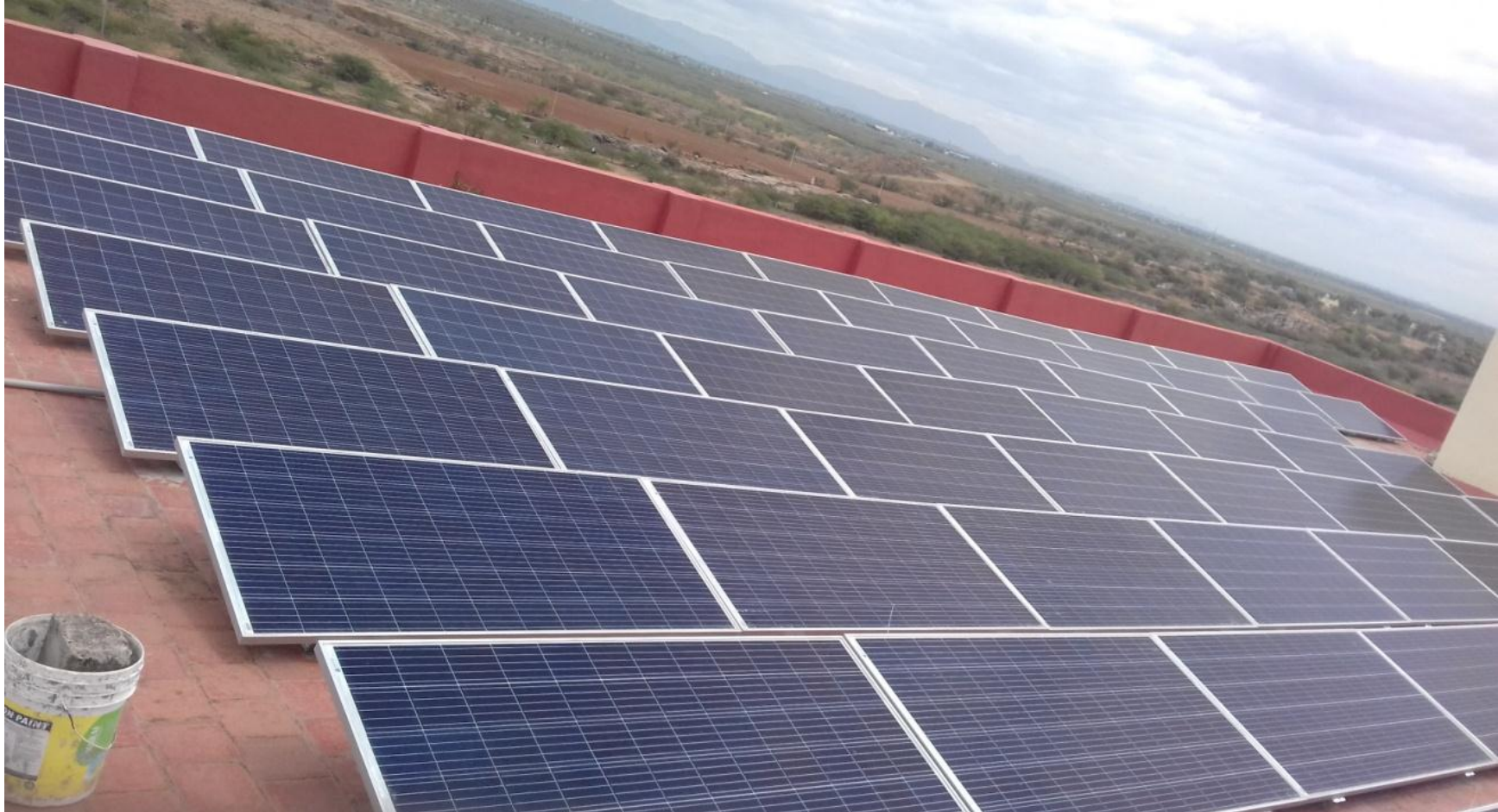
Solar panel placed in top of the EEE Department
